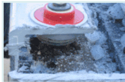
<Battery terminal deflection >
